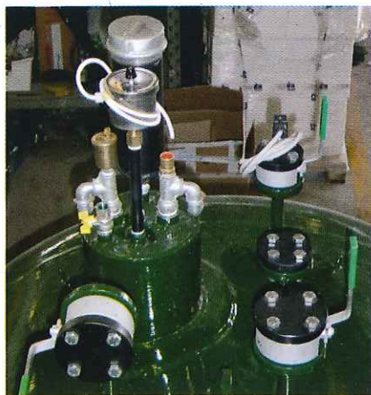
Instruments and accessories for control of the heat exchanger
