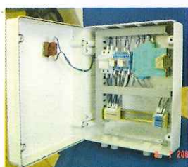
Electric Panel with Zener barrier
